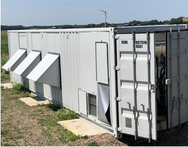
Figure 1: Photo of the presented FRT Testsystem for UVRT and OVRT Compact in one standard ISO 40 foot container
