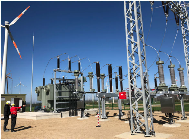
Figure 6: Outdoor substation components for High Voltage Test System
