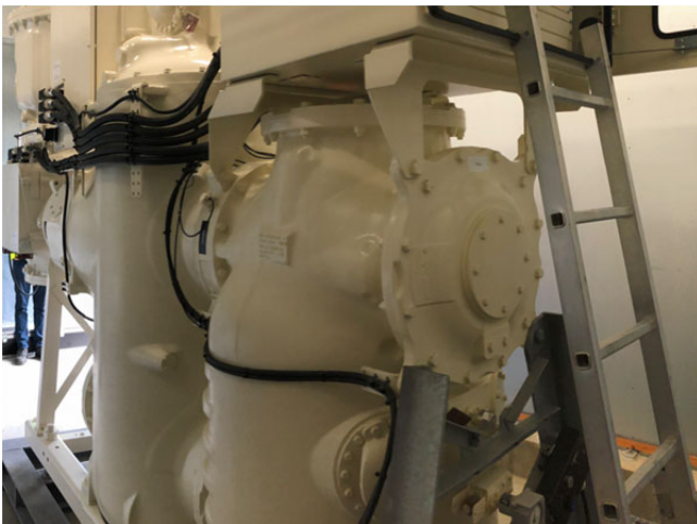
Figure 7: SF6 Gas isolated switch gear components for High Voltage Test System
